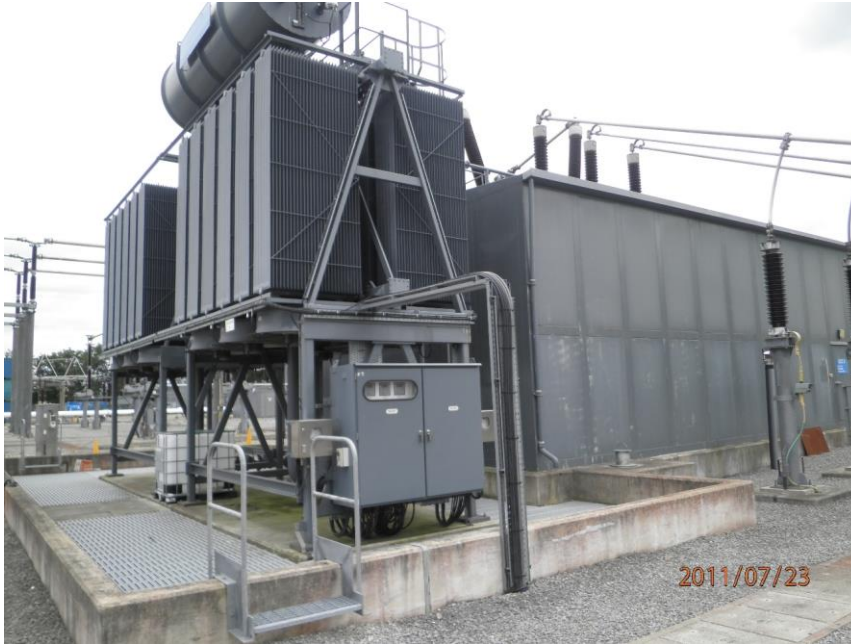
Plate 4.9 Typical (large 400kV) power transformer
