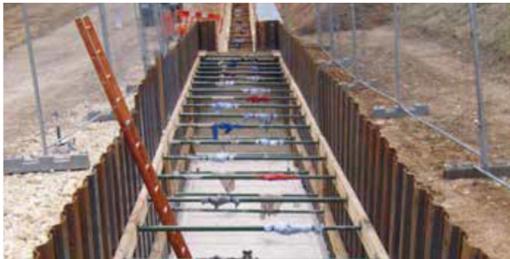
Plate 4.10 Typical Joint Bay
